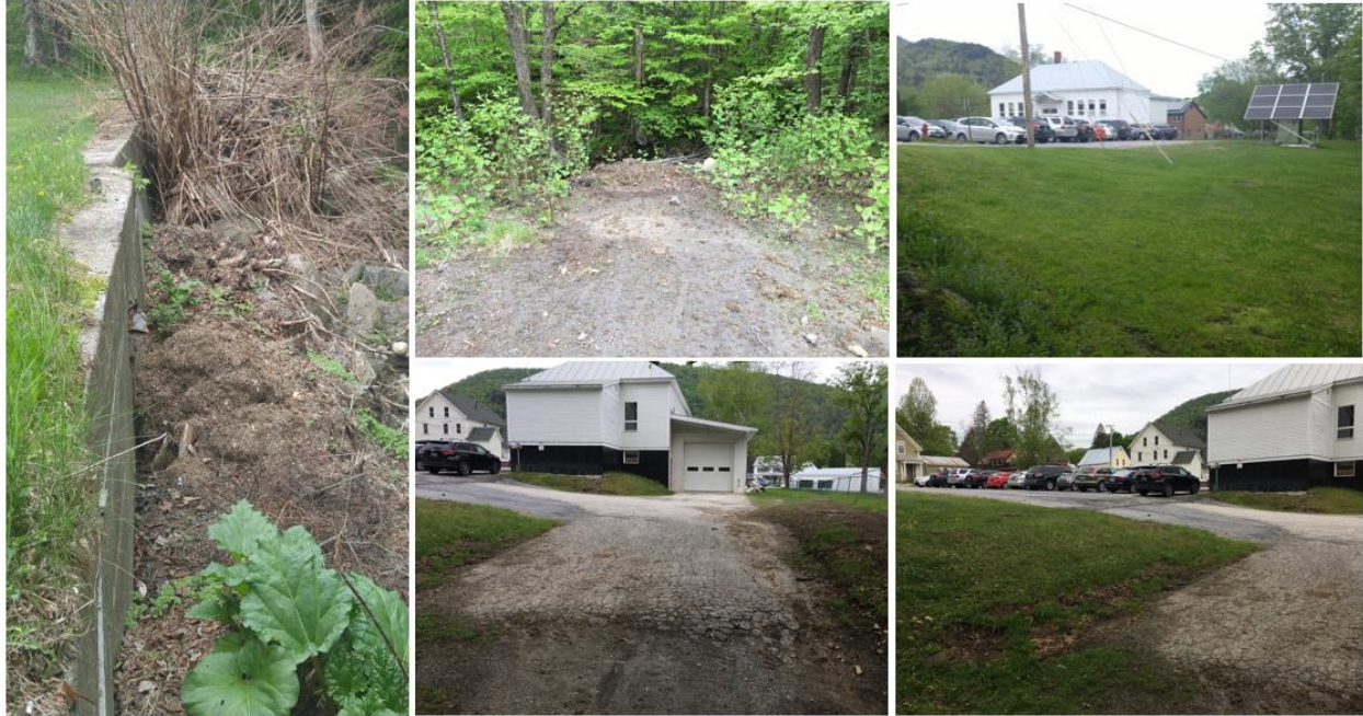
Figure 8. Image on the left shows the stream bank with lawn waste material and no vegetated buffer at the stormwater discharge point. Other photos illustrate the view from the edge of the parking lot looking toward the stream with indication of stream bank erosion and signs of winter snow storage and the mown grassy lawn adjacent to the waterbody. The proposed practice would be placed in the current snow storage location (shown in the bottom two images above).
